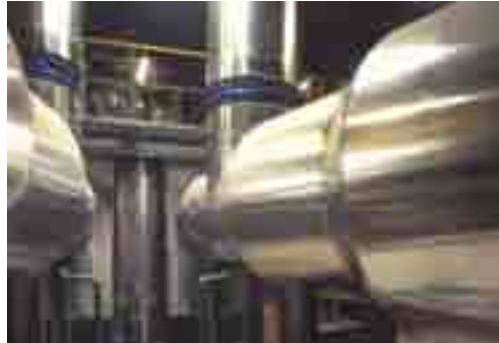
Cogeneration plant in Castelvetro
